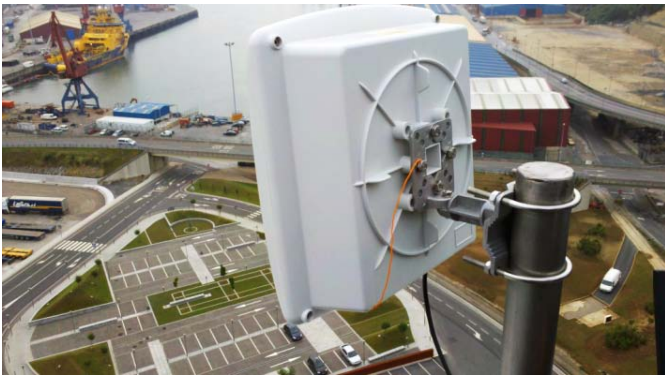
Figure 6. Device deployed inside an antenna case on Bilbao's harbor controlling railway signaling over a dedicated WPAN.
